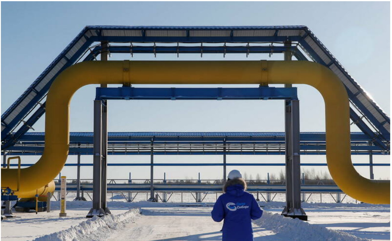
An employee in branded jacket walks past a part of Gazprom's Power Of Siberia gas pipeline at the Atamanskaya compressor station outside the far eastern town of Svobodny, in Amur region, Russia November 29, 2019. (Maxim Shemetov./REUTERS)
